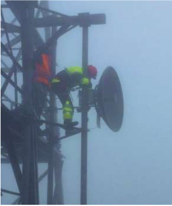
Fig. 8 Antenna at the tower in Mount Limbara
